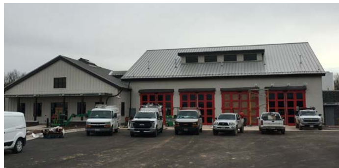
Loudon County Lucketts Fire & Rescue Station, currently under construction and designed for green building certification
